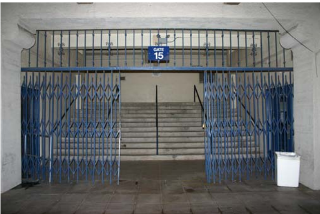
Entrances to steps and the 2 nd floor have rickety, old metal gateways that are closed and locked between 5PM and 8AM, making entry/exit difficult for staff and faculty after hours, and a hazard in case of emergencies.
