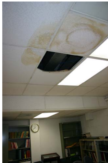
Chronic leaking through the concrete bleachers overhead repeatedly ruins ceiling tiles and damages research and teaching materials in our offices and labs.
