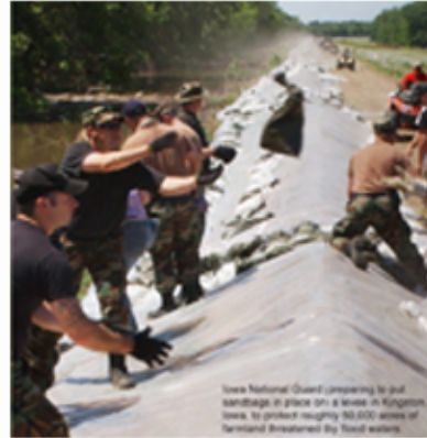
Iowa National Guard preparing to put sandbags in place on a levee in Kingston, Iowa, to protect roughly 50,000 acres of farmland threatened by flood waters. Source: Iowa National Guard photo by Sgt. Chad D. Nelson
