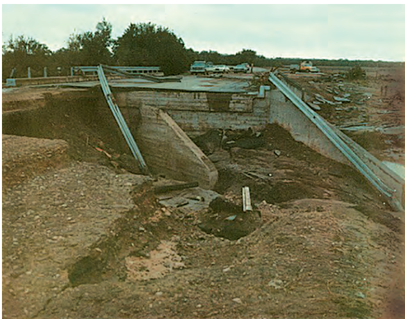
Figure 6. View of right end of bridge across North Fork Hubbard Creek near Albany, Texas, August 1978. Flow was about 2 feet above guardrails.
