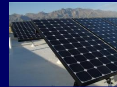
Photovoltaic (PV) panel
